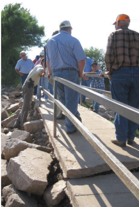
Stuart Schrag shows damaged ramp to CMC in August.
